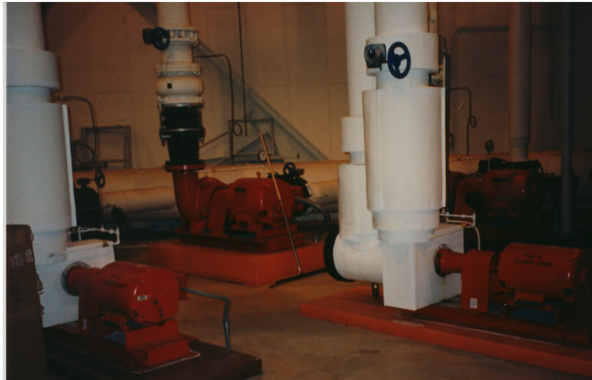
Figure 3-4: Example of good thermal insulation in a chilled water system (Observe that chilled water pumps, valves and pipes are all well insulated)
